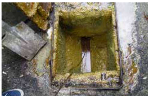
Food premise manhole with evidence of FOG
