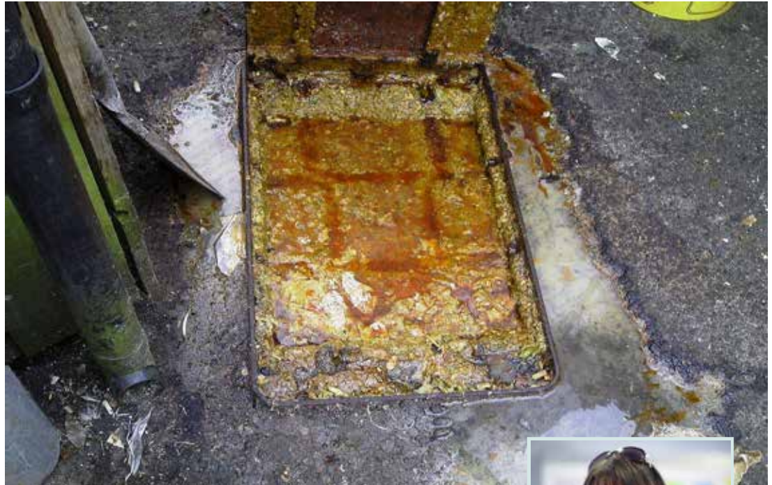
A manhole full of Fats, Oils and Grease
