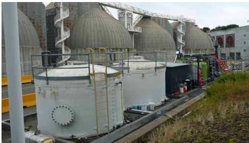
The FOG to biodiesel pilot plant at Oceanside WwTW with the digesters in the background.
